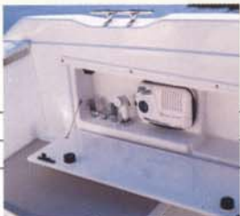
Transom Shower and Air Compressor
