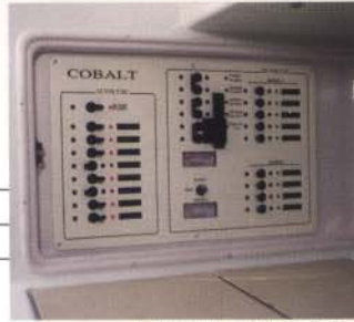
AC/DC Distribution Panel
